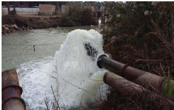
Fig. 6. The pump station of AlMahawil stream with operation of 3 m 3 /s (Directorate of Water Resources in Babylon, 2019)
